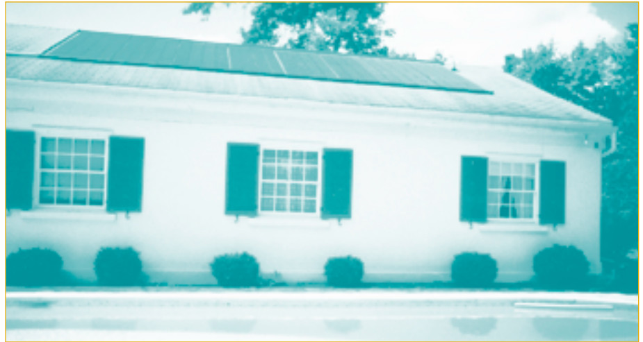
▲ Ottawa, Ontario. 6.1-m x 12.2-m (20-ft. x 40-ft.) in-ground pool, eight 4.4-m 2 (4-ft. x 12-ft.) solar collectors. Photo courtesy of Heliocol Canada.
