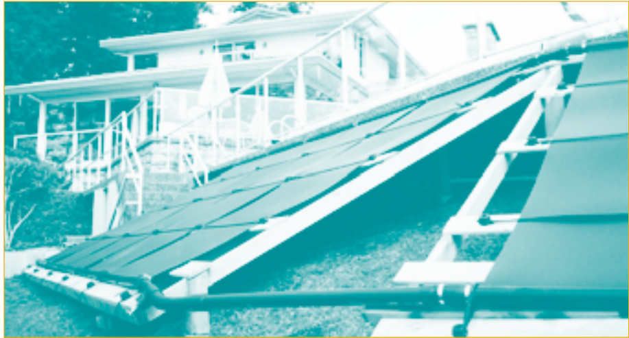
▲ White Rock, British Columbia. Eight 4-m 2 (4-ft. x 10-ft.) solar collectors on a wooden ground rack. Photo courtesy of Taylor Munro Energy Systems.
