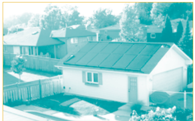
▲ Welland, Ontario. This 5-m x 10-m (16-ft. x 32-ft.) free-form pool is heated by six 4.4-m 2 (4-ft. x 12-ft.) solar collectors mounted on the garage. Photo courtesy of Daystar Energy.
