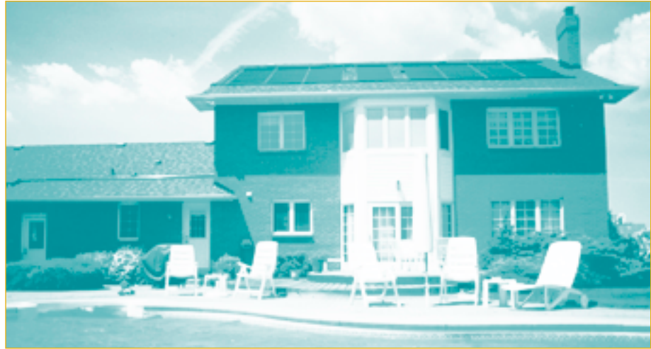
▲ Fonthill, Ontario. This 6.1-m x 12.2-m (20-ft. x 40-ft.) pool has a solar cover and eight 4.4-m 2 (4-ft. x 12-ft.) solar collectors. Photo courtesy of Daystar Energy.
